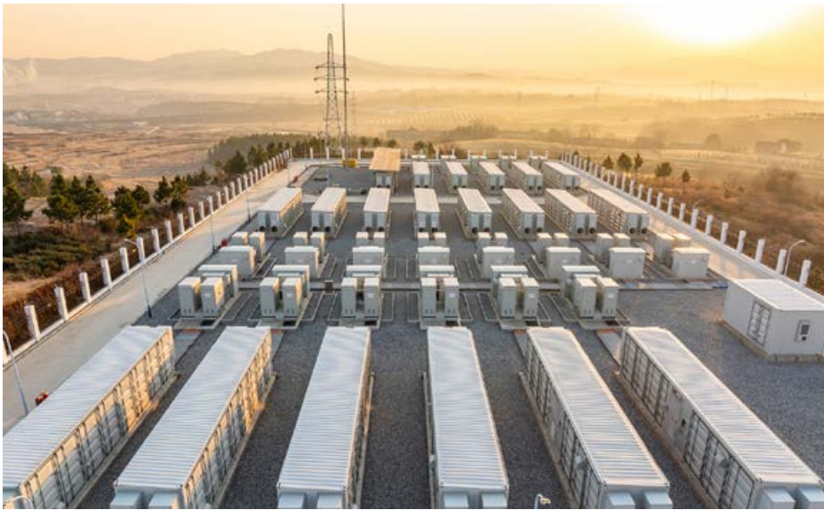
Power play Battery storage is in demand
