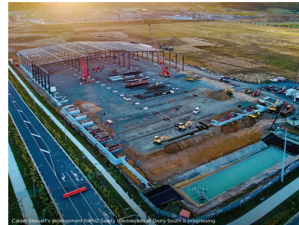
Calder Stewart’s development for NZ Safety Blackwoods at Drury South is progressing
